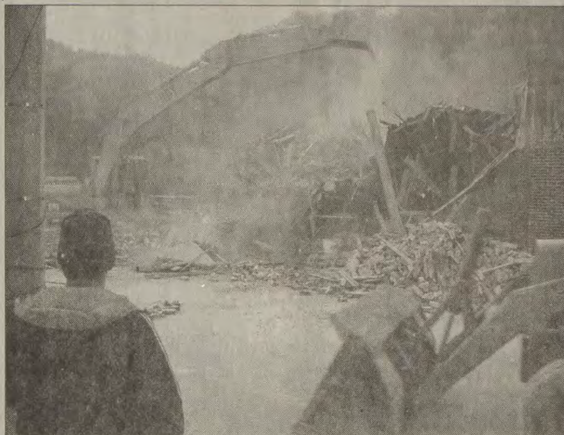
photo by Tom Doty The old Prestonsburg Hospital, which has most recently served as offices for Mountain Comprehensive Care, was demolished Tuesday evening. Mountain Comprehensive Care recently constructed a new office building at the site of the old Hobb's Five and Dime.
