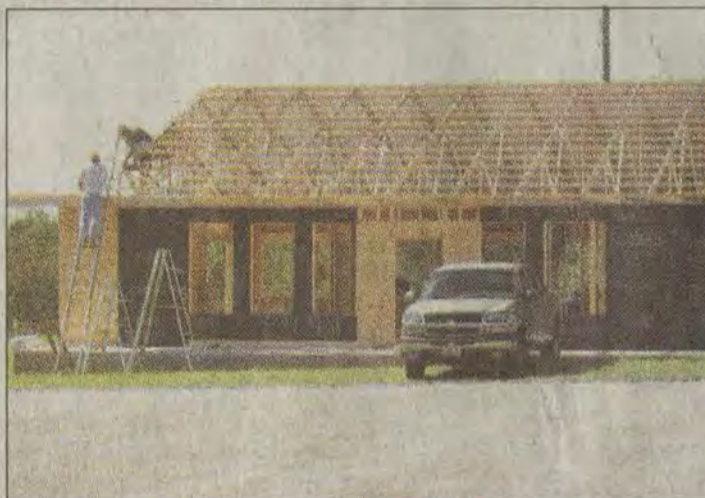
Cloud Nine Restaurant, currently under construction, plans to serve meals to both airport and prison traffic, as well as any other businesses which locate in the Honey Branch Industrial Park.
