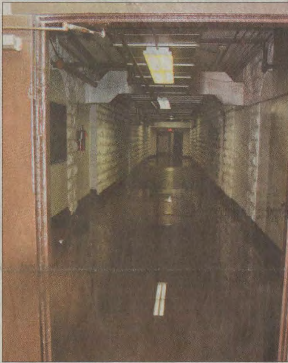
Steady rains overnight Wednesday forced Prestonburg Elementary to evacuate its basement due to flooding. School officials said at the time that basement flooding during rainy periods has been a chronic problem of late.
