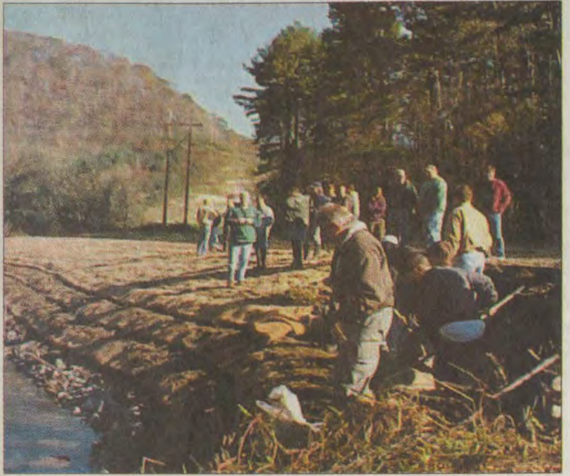
Participants in the soil bioengineering workshop are shown installing soil blankets and layers of willow cuttings between the soil blankets.
