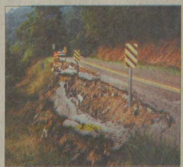
Residents of Abbott Creek who travel Route 1750 near Bonanza have had to contend with a dangerous break in the middle of a double-blind curve since February. Several have expressed outrage that the problem has not been fixed, despite the obvious danger it poses.
