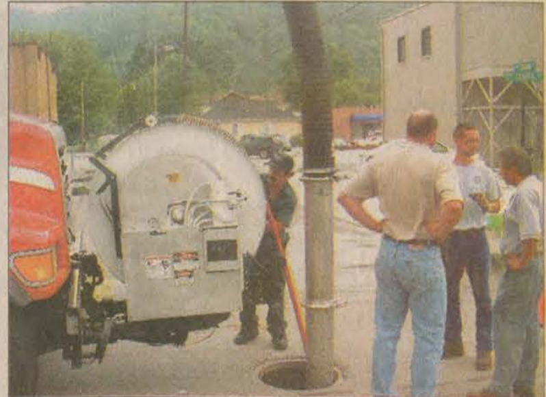
Prestonsburg city utility workers used the new "Sewer Vacuum" on South Central Avenue on Wednesday. Workers hope that the new machine will help curb the city's sewage odor problems.
