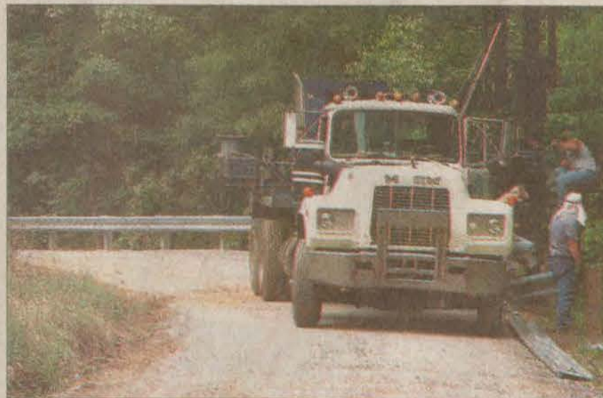
A guardrail is under construction in Galveston in an effort to prevent accidents and increase the safety of the road.
