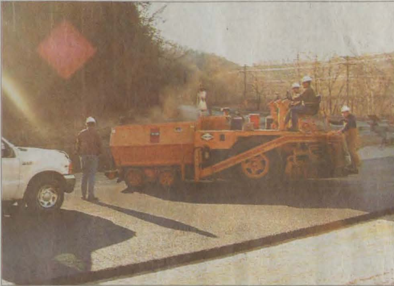
Construction workers spent Wednesday afternoon paving the northern entrance to Jenny Wiley State Resort Park. photo by Sheldon Compton
