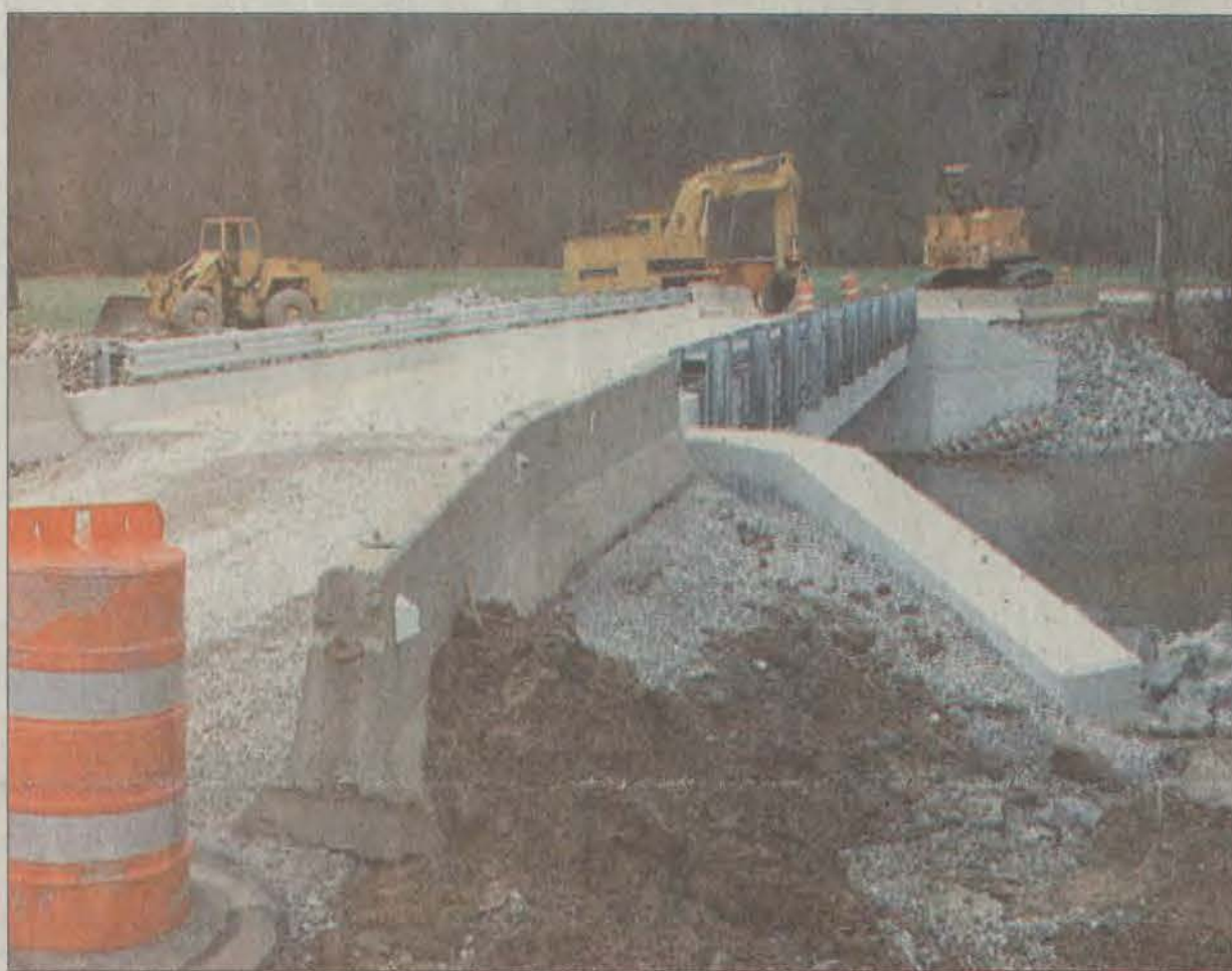
At Granny Fitz Branch, work on a new bridge which serves as the road's only connection with the outside world is mostly completed. In December, a county truck carrying blacktop collapsed the old bridge, requiring a makeshift span to be erected until the replacement could be built.
