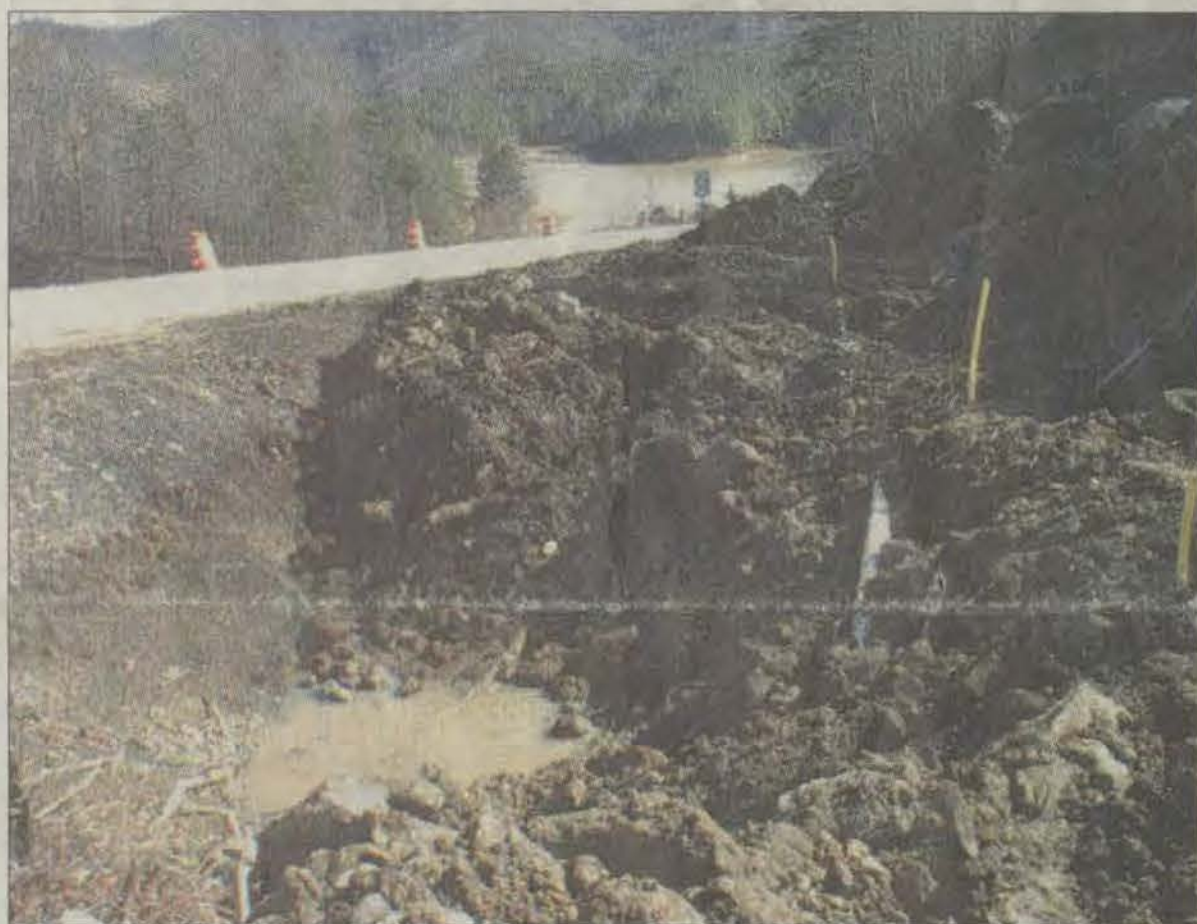
Another damaged line left Lake View Village residents without water again this week. The break was due to a miscalculated blast during construction at Dewey Lake Monday evening.
