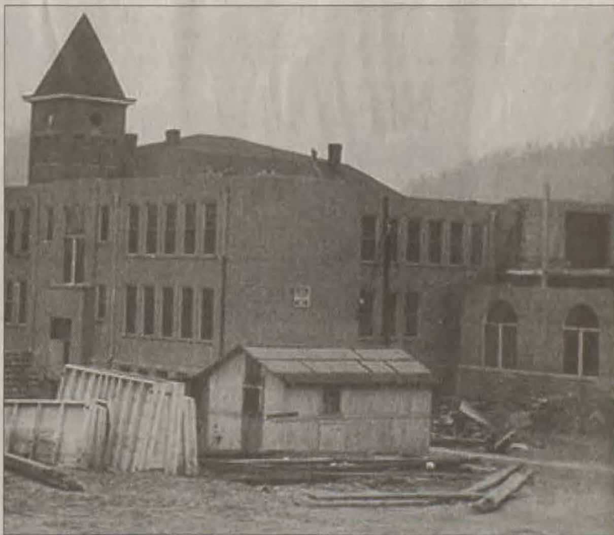
This shows the present-day Prestonsburg Elementary School during the period when it was being constructed. It was erected on the site of the old Baptist Institute, the upper part of which can be seen here. The Baptist Institute served as the town's high school and grade school during the 1920s and was still being used when this photo was taken. At right is the PHS gymnasium. Photo courtesy of the Kentuckiana Archive of the Kentucky Virtual Library at www.kyvl.org
