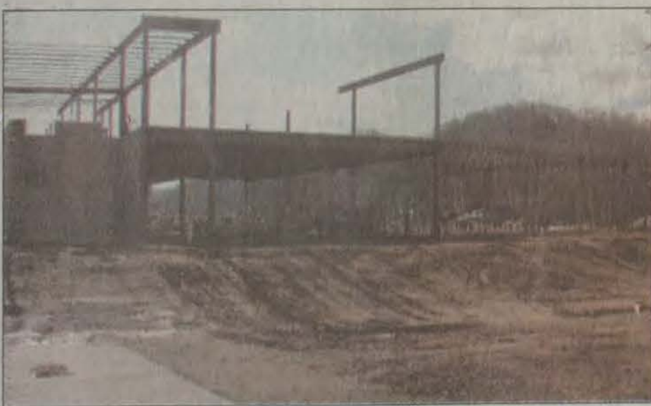
Early construction efforts have gotten underway at Prestonsburg Community College on what will soon become the site of three educational additions, including a state-of-the-art planetarium that will serve the community as well as students once completed. The building shown will serve as a classroom building, as well as the school's new student center.
