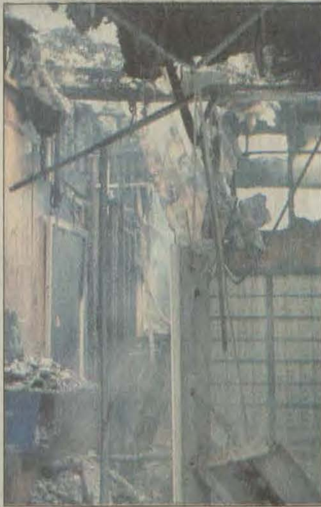
Flames left the interior of the Bypro Post Office in shambles as portions of the collapsed roof dripped with burning ash covering what was once the front office.
