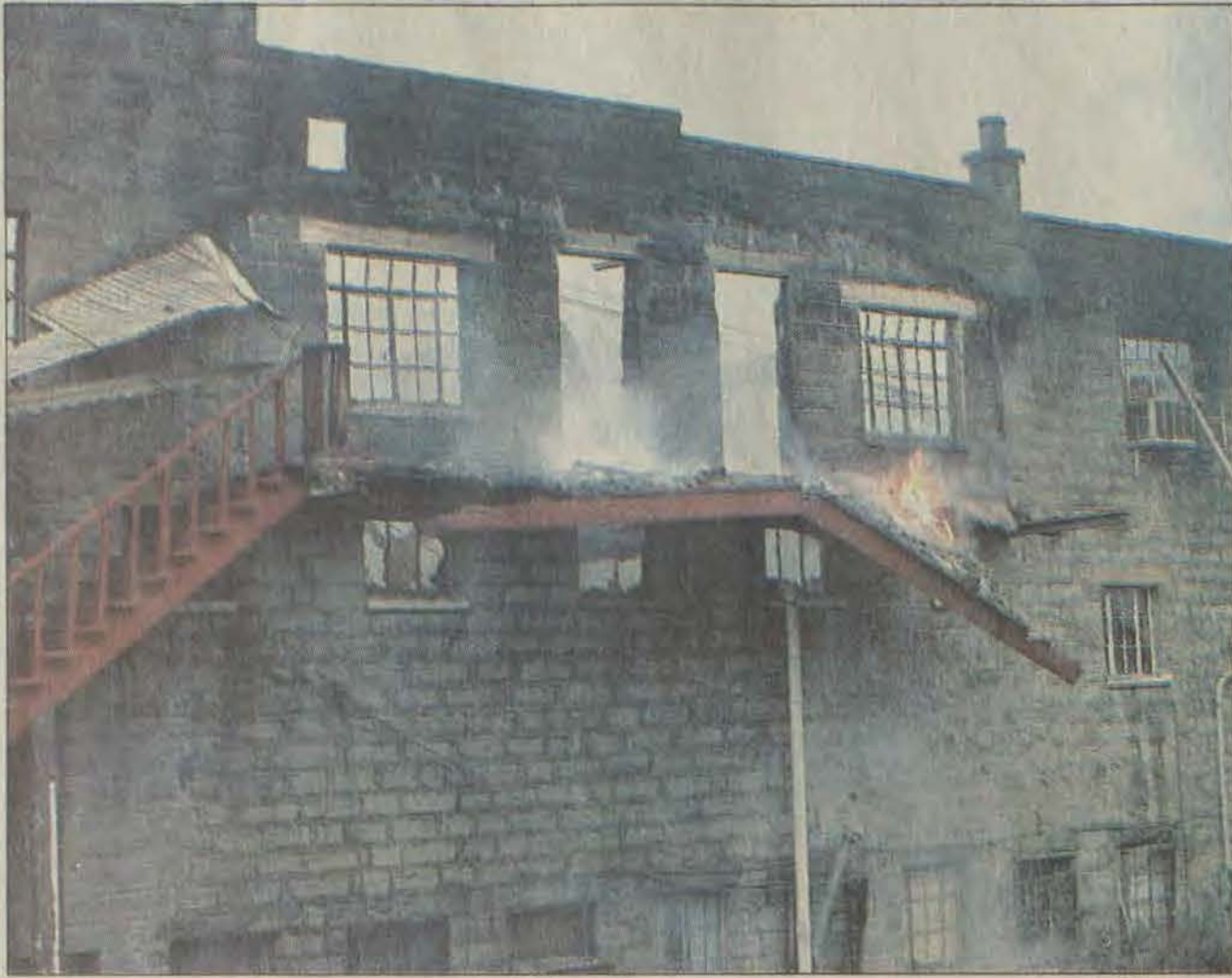
All that remains is an empty stone structure as an awning along the side of the Bypro Post Office building threatens to break away as flames extend from an upstairs window.
