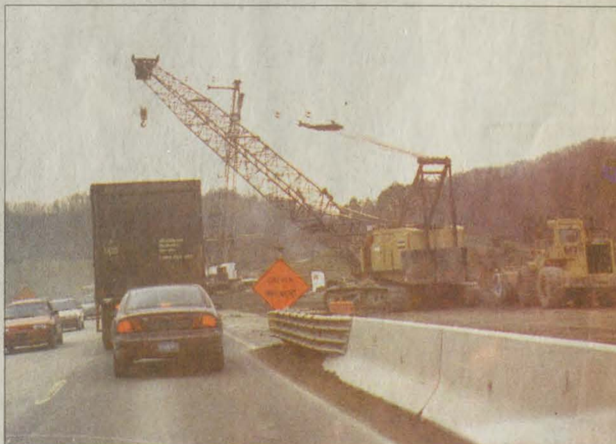
Motorists on KY 114 found it necessary to drive under the arm of this huge crane for a short time last week. The crane is used in the construction of a bridge located near the Mountain Arts Center. (photo by Willie Elliott)
