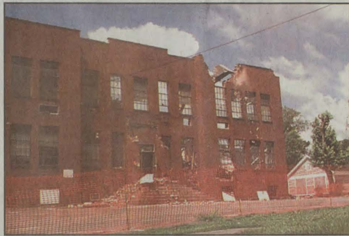
The former offices of the Floyd County Board of Education came crashing down Friday and Saturday. The board moved from the former school building earlier this year and now occupies the former Bank Josephine building on Front Street in Prestonsburg.
