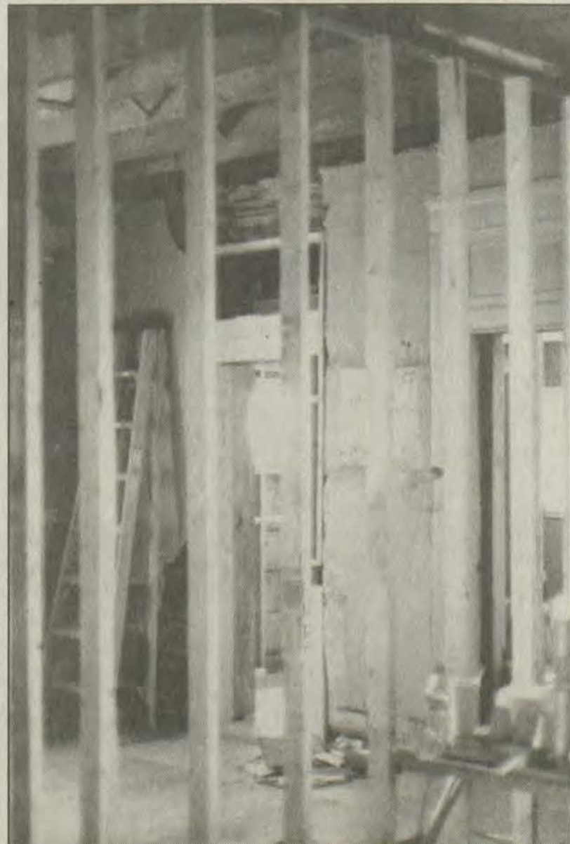
Faulty wiring and plumbing, termites, and the forces of age meant extensive reconstruction needed to be done on the South Lake Drive house, which has been turned into offices for the Ramey Insurance Agency.
