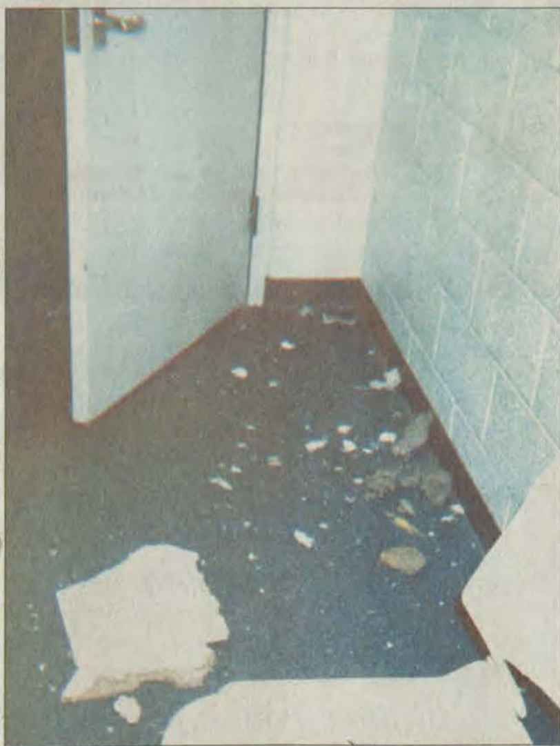
During blasting associated with widening KY 114 a rock came through the roof of the Mountain Arts Center (MAC). Director Kevin Shannon said the foreman from Bizzack, the construction company doing the road work, was on hand immediately to survey the damage. The roof has been patched, but Shannon said the whole panel would have to be replaced. The MAC has a metal roof.
