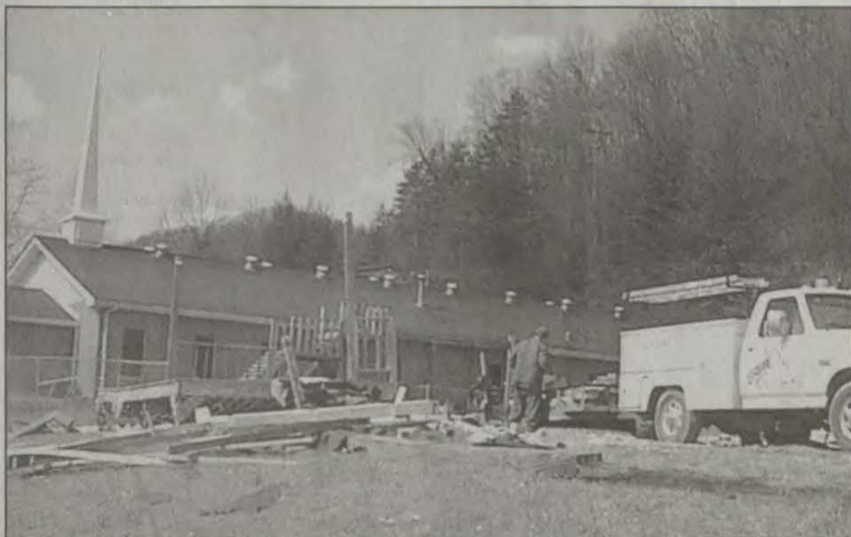
The parsonage at the Fitzpatrick Baptist Church on KY 114 was moved Thursday. The church is next on the demolition block. A four-lane highway will replace the church. The Fitzpatrick Baptist Church congregation is building a new church at Big Branch of Abbott Creek. They will conduct special services this weekend. (photo by Janice Shepherd)
