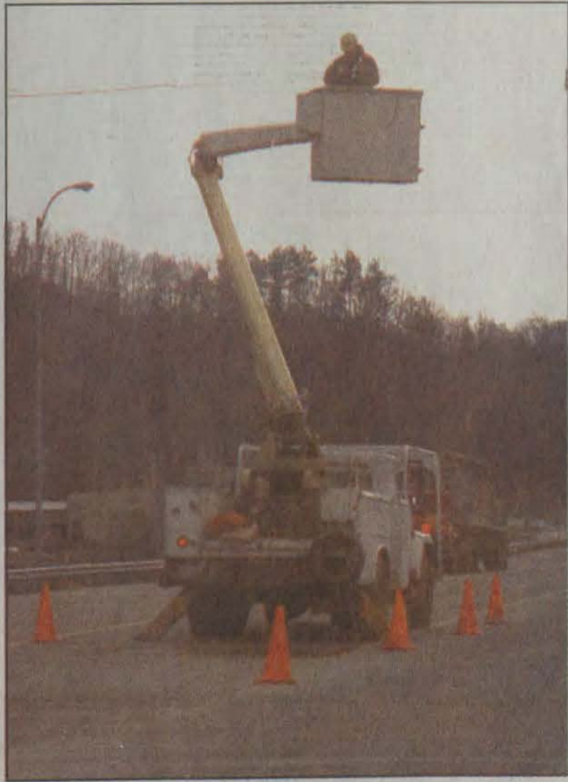
On Monday afternoon Joey Ratliff with Davis Elliott Contractors was high above the traffic on KY 80 installing one of the traffic lights at the Lancer-Watergap cloverleaf where KY 80 and US 23 meet. This makes two sets of lights at this location. At presstime highway officials did not know when the new lights would be in operation. (photo by Willie Elliott)
