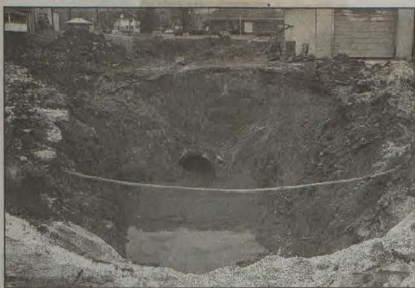
'There's a hole, there's a hole ...' Bob White Construction Company created this huge hole as a drain pipe was replaced on West Friend Street in Prestonsburg. The street near First Commonwealth Bank has been closed as the company finishes the work. (photo by Willie Elliott)
