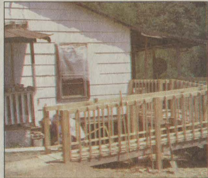
Melissa Ross and Rev. Dave Diamond are almost hidden by the large ramp they helped build on a Jack's Creek residence as they work on underpinning the house. They and other members of Utica United Methodist Church in Sterling Heights, Michigan, were here last week on a working vacation, volunteering through the Appalachian Service Project. (photo by Pam Shingler)
