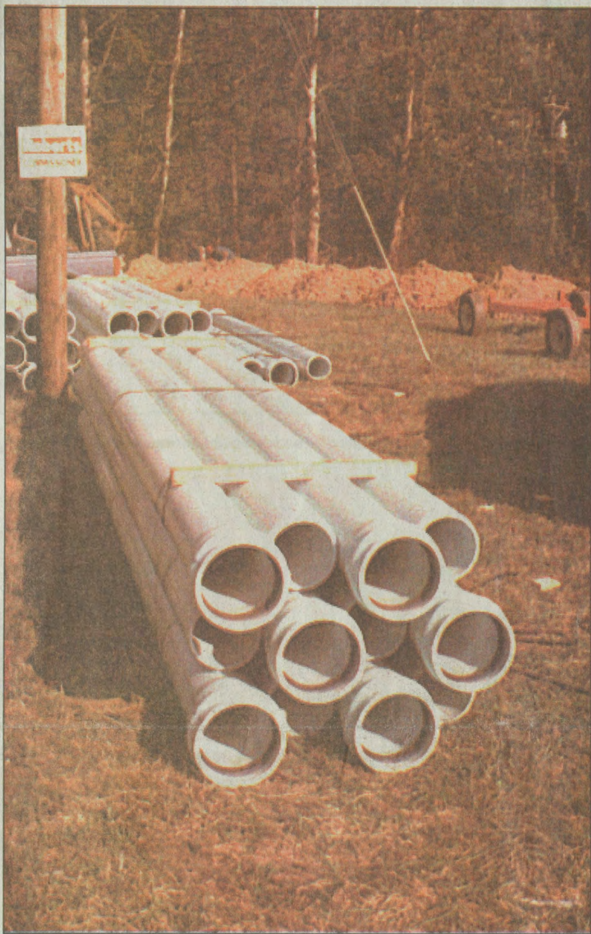
Water and gas lines are being moved for widening of a two mile-stretch of KY 404 to U.S. 23 and KY 114, an extension of the Mountain Parkway. Four-laning of the road from Prestonsburg to Salyersville should be completed by 2004, transportation officials said this week. (photo by Ed Taylor)
