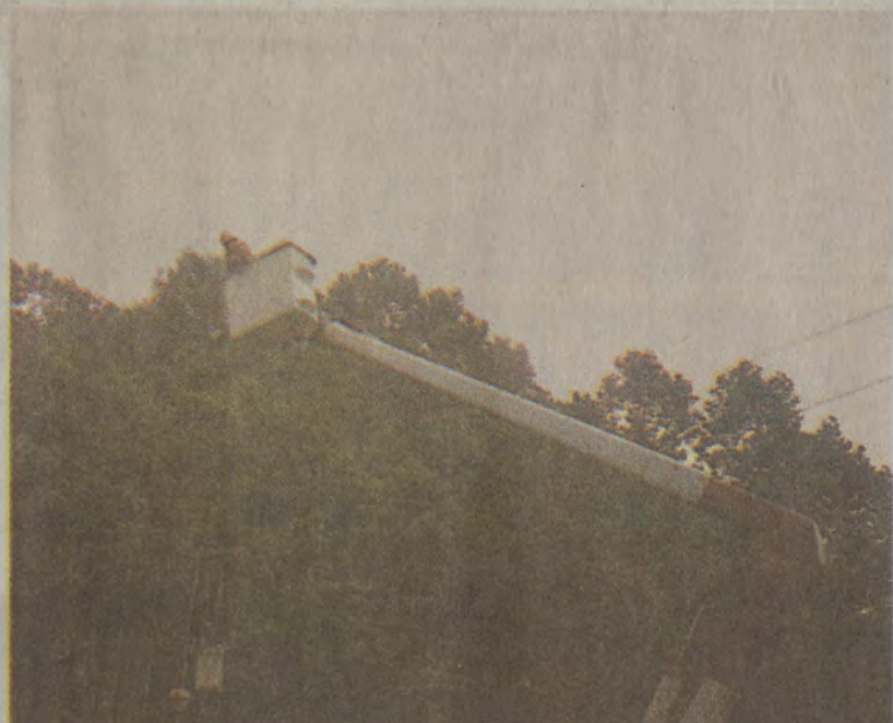
Wednesday was not the greatest day for a resident of the right fork of the Little Paint area, as Ricky Setser captured on film the aftermath of the storm damage to neighbor Bill Vaughn's home, where a tree fell. Here, a power crew works to repair lines. (photo by Ricky Setser)
