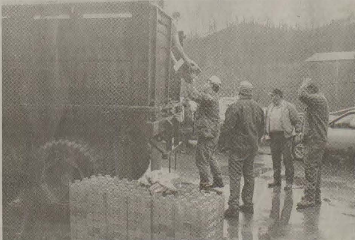
The National Guard shipped in 16,000 gallons of water Wednesday afternoon to Beaver Elkhorn Water District customers. A water line break has left hundreds in the Right Beaver area without water. Efforts to repair the line have been hampered because the damaged line is under flood waters. (photo by Chris McDavid)
