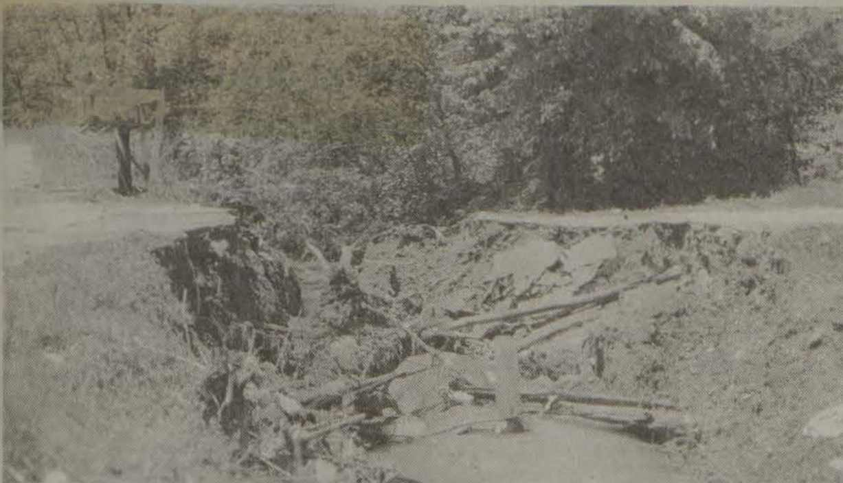
Flood waters wash out access road
