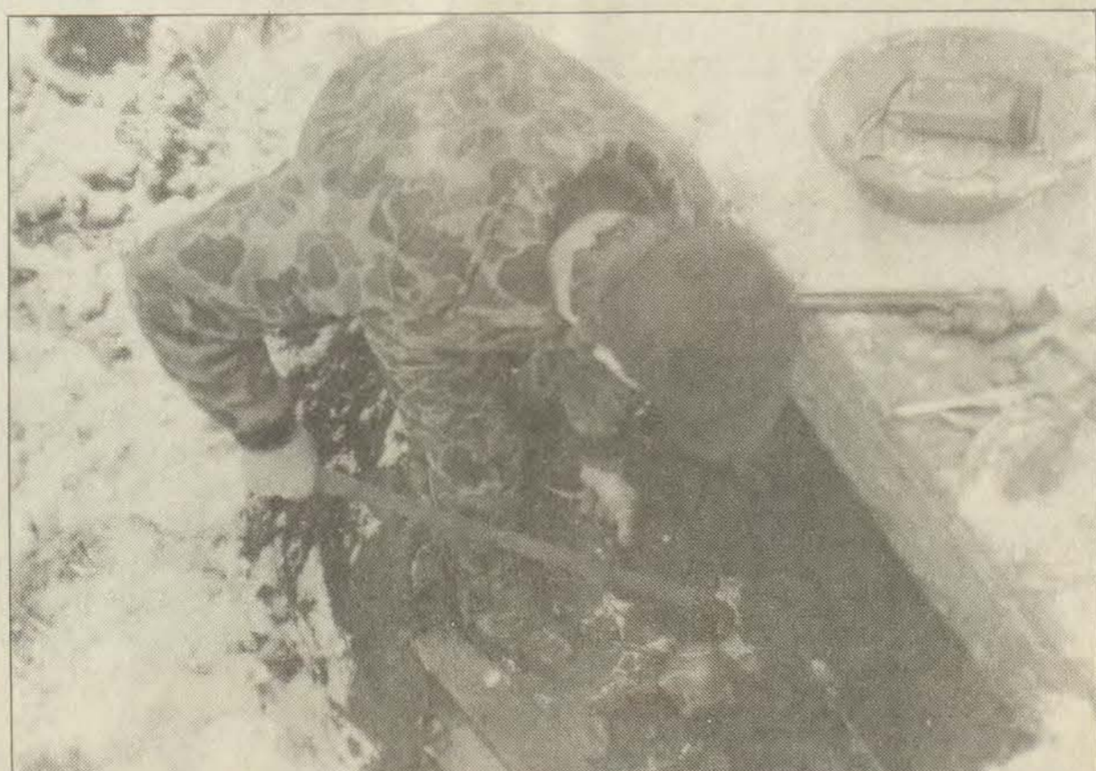
A Bundle Of Busted Pipes
