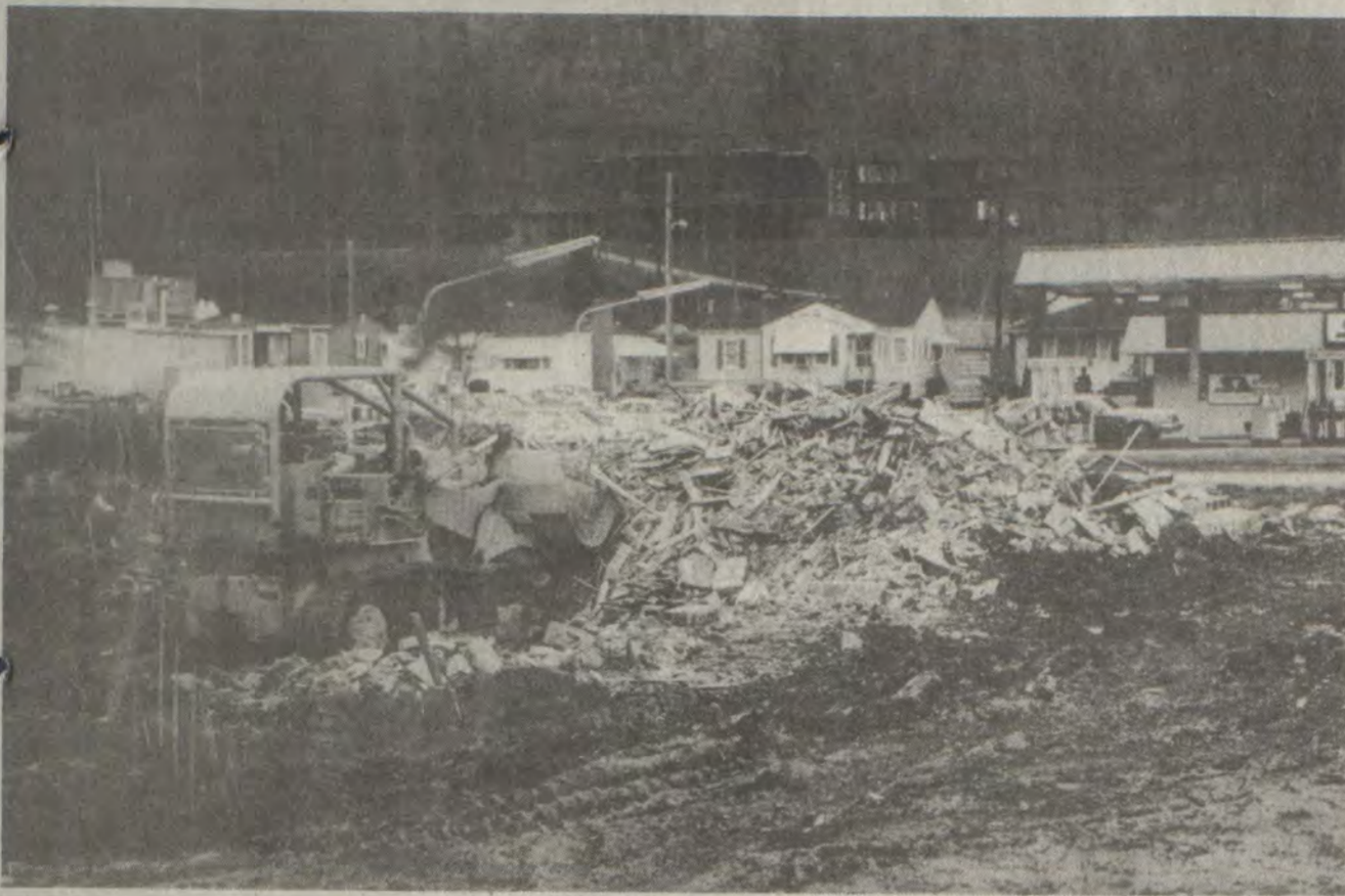
HERE TODAY, GONE TOMORROW: The home at 426 N. Lake Dr. disappeared overnight last week, and most of the motel next door was gone by the next afternoon. Ed Kuss, who owns both pieces of property, said he plans to build a Taco Tico on the site. Serving authentic Mexican food, the full-service, fast-food restaurant will be "a fancy, pretty place that Prestonsburg will enjoy and will add to the area," Kuss said.
