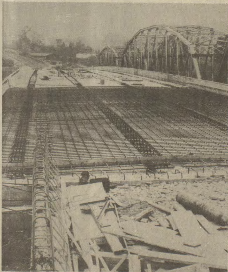
NO WORK HAS BEEN DONE on the new bridge over the Big Sandy at Allen since the construction firm, C&C Contracting, of Williamsburg, defaulted six weeks ago. A new contractor is being sought by the bonding company, which now is responsible for seeing the job completed. The $2.3 million project, now 70 percent complete, was supposed to have been finished by the end of this month.
