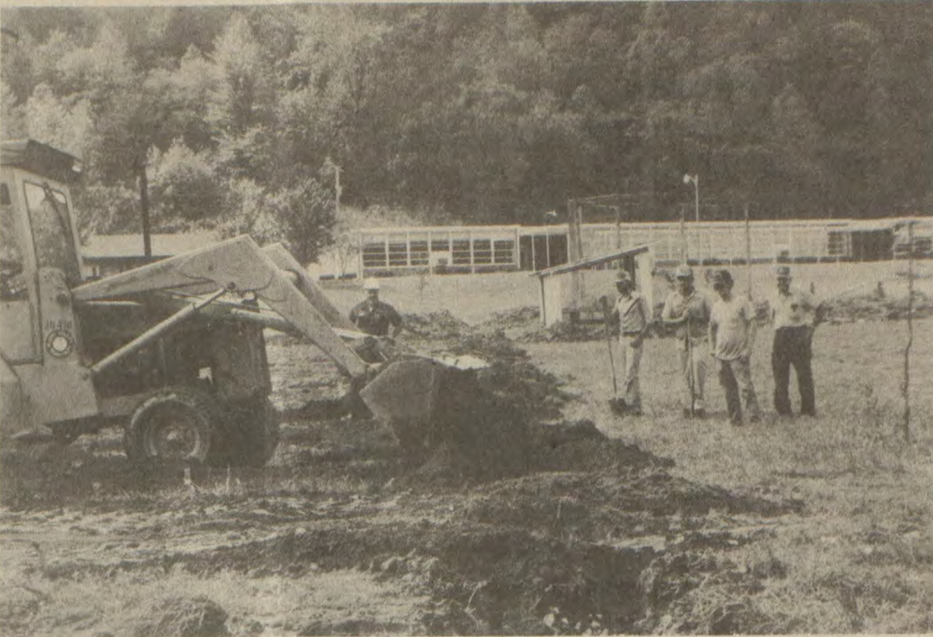
THE BALLFIELD at Clark Elementary School, plagued by a drainage problem, should be drier from now on as the result of a joint effort among U.S. Soil Conservation Service technicians, county laborers, and the Floyd County Conservation District. A 600-foot drainage tile was being covered when this picture was taken Thursday. A drainage ditch is also being constructed at the foot of the hill behind the school.
