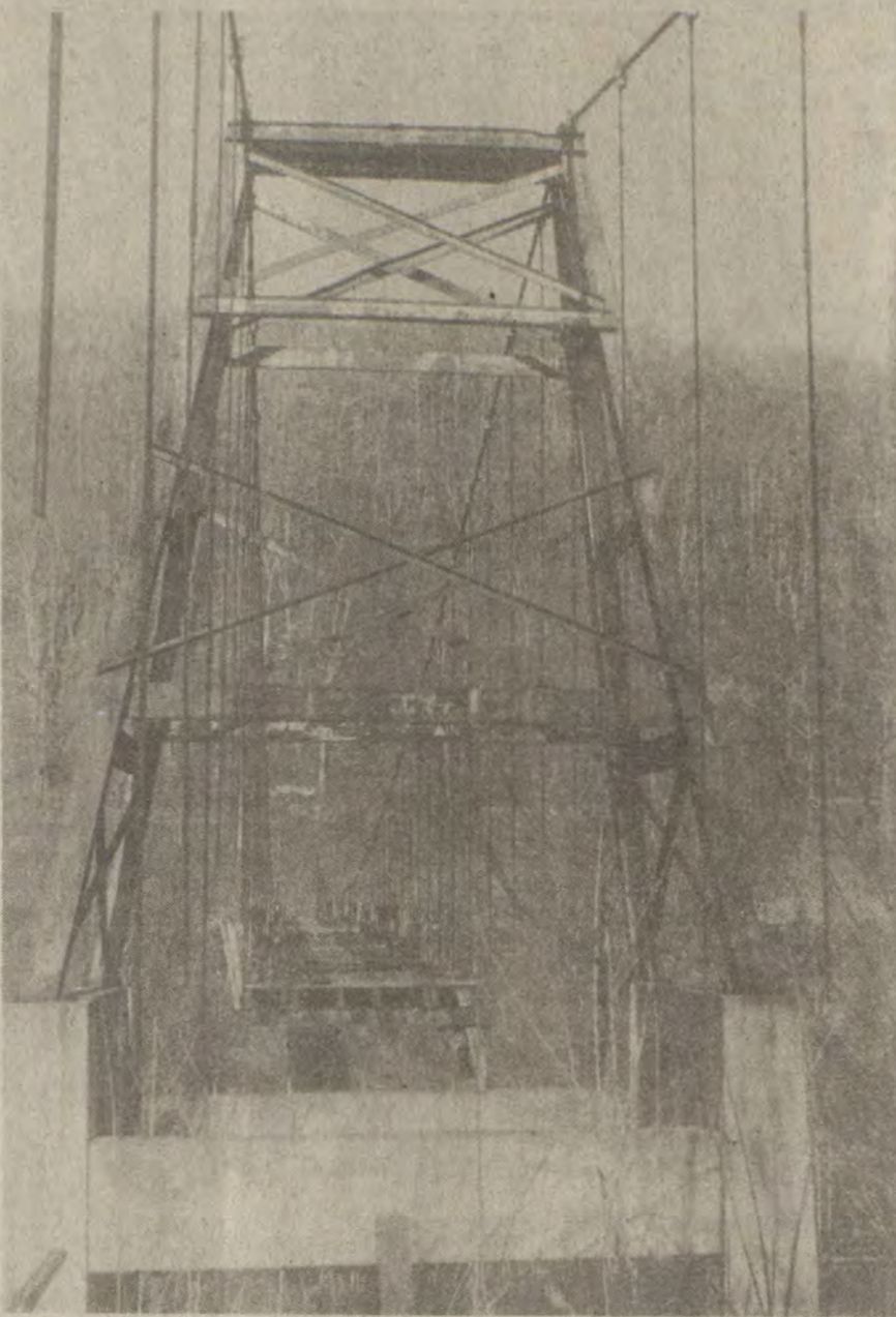
TENUOUS STRANDS of this long-disused suspension bridge over the Big Sandy at Knotley Hollow are destined for the junkyard. A contract for replacing the structure, which once provided access to residents of the Goble Roberts Addition from KY 1428, could be let as early as next month. A two-lane concrete span is proposed, at an estimated cost of $1.1 million.
