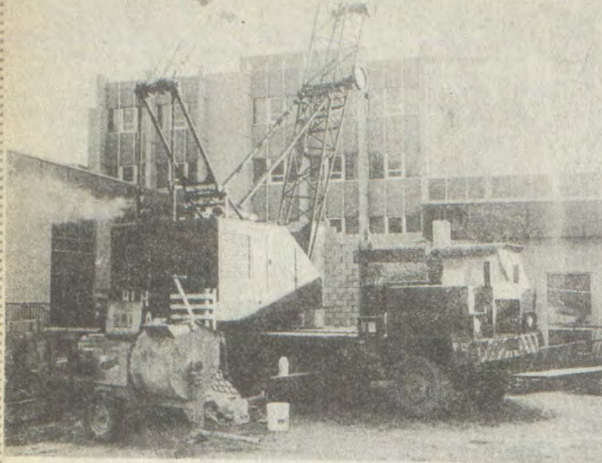
A crane waits to install the elevator in the new entrance to ground floor medical offices at HRMC.
