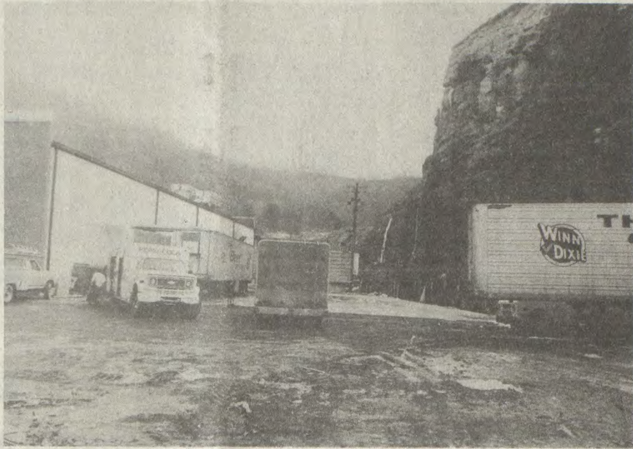
WHOLESALEMADE deliveries last week under the shadow of the highwall that rises behind newly-opened stores in the Prestonsburg Village shopping center. City building code officials have warned that the cliff face is unstable and hazardous and have ordered developers of the shopping center to take steps to stabilize it. Developers said they were bringing in equipment this week to remedy the problem.
