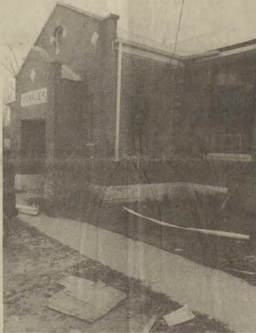
DEBRIS, including guttering that has fallen from the eaves, litters the grounds of the 44-year-old Dwale schoolhouse, which has been for five years the site of Floyd county's only class for multi-handicapped children. But more worrisome even than the debris, for parents of the seven youngsters enrolled there, is their children's isolation from their non-handicapped peers.
