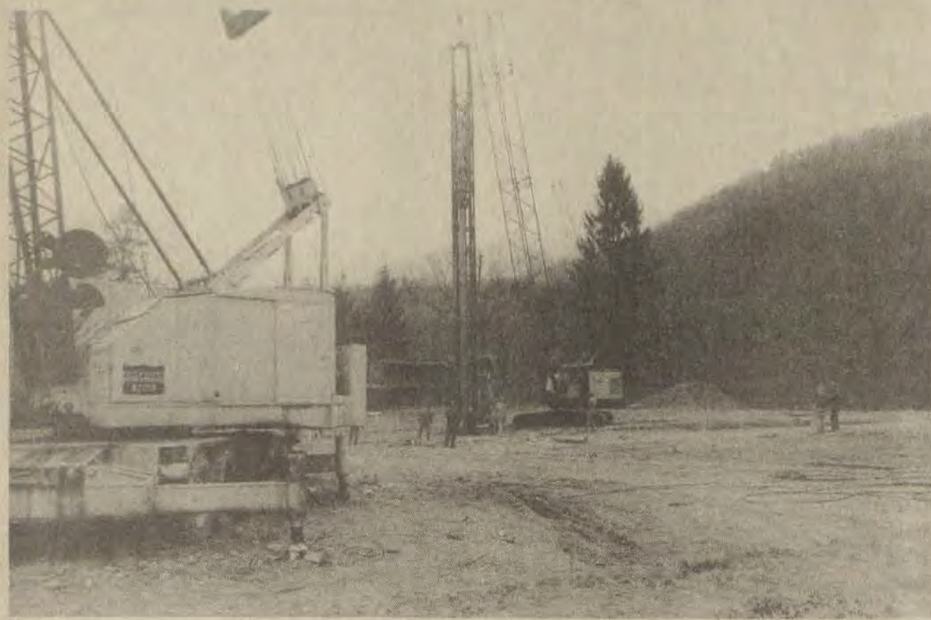
WITH SITE PREPARATION and clearing work complete, first stages of actual construction began this week on First Commonwealth Bank's new multi-million facility. Located on the former Garfield Place property and adjacent lots on Arnold Avenue here, the five-story structure will provide 78,000 square feet of space and will contain all departments of the bank that are now housed in the First Commonwealth building at the corner of Court Street and Lake Drive. Akers & Akers are contractors on the $6.5 million project.
