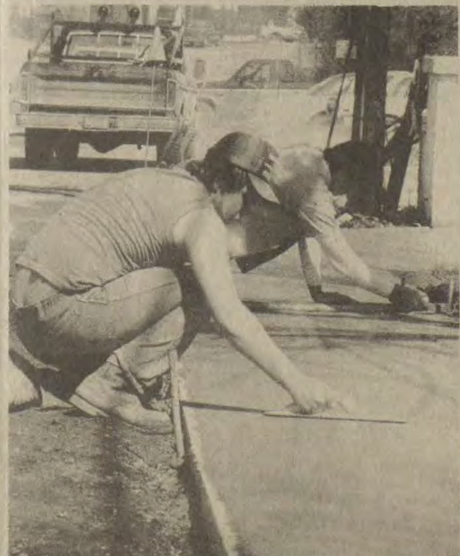
SIDEWALKS were being poured, Tuesday, along a section of old KY 80 near Our Lady of the Way Hospital at Martin. Work is being done by Burton Concrete Construction, a Johnson county contracting firm.
