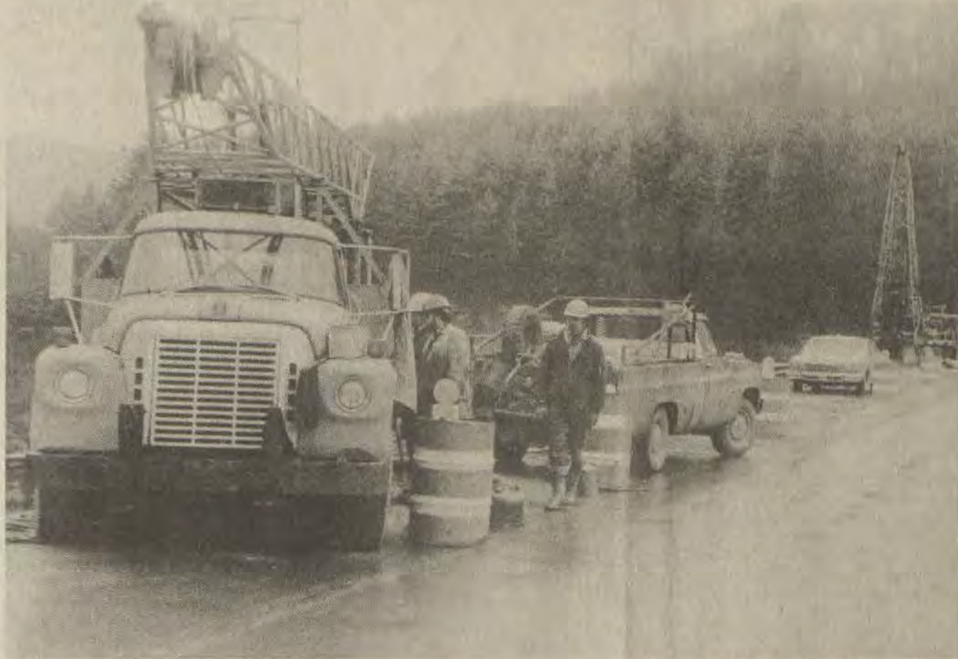
CORE DRILLING EQUIPMENT of the Mott Drilling Company, of Huntington, W. Va. was being used last week to take soil and fill samples from Dewey Dam, one of a number of work projects currently underway there. From the core samples, geologists will determine such factors as soil and material density and permeability. In addition, several pizometers, instruments for accurately gauging water levels underground, will be installed in selected test holes. Similar testing and instrument installation will be made at the dike at Brandy Keg, according to Dean Murray, Corps of Engineers reservoir manager.
