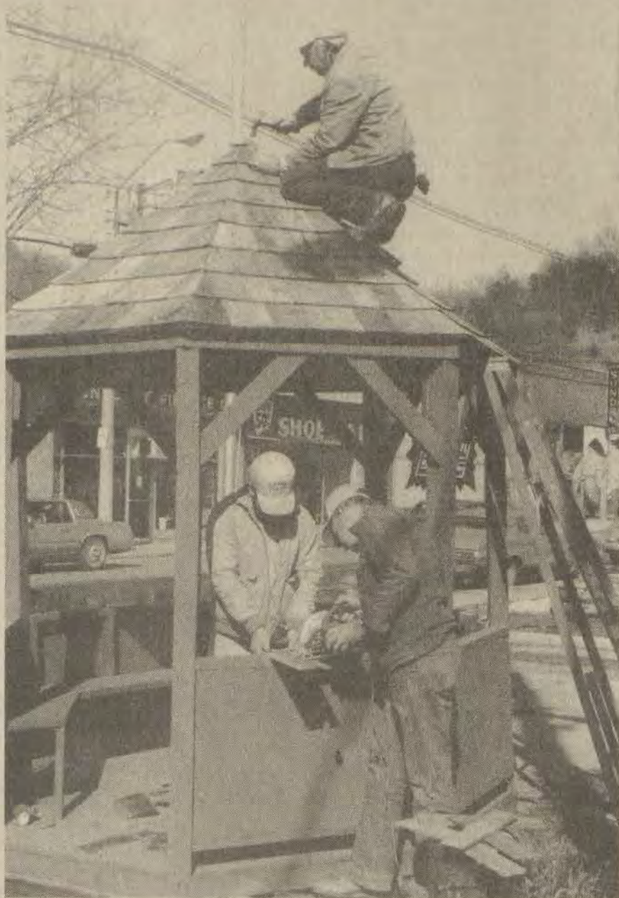
IT WAS A BRIGHT, sunny day (for a change) last week when this photo was snapped of a crew of city employees adding finishing touches to a cedar, gazebo-like structure at the municipal parking lot on Court Street here. Roofed and provided with benches, it should make a nice rest stop for weary pedestrians or an ideal place for a bit of whittling on a rainy day.
