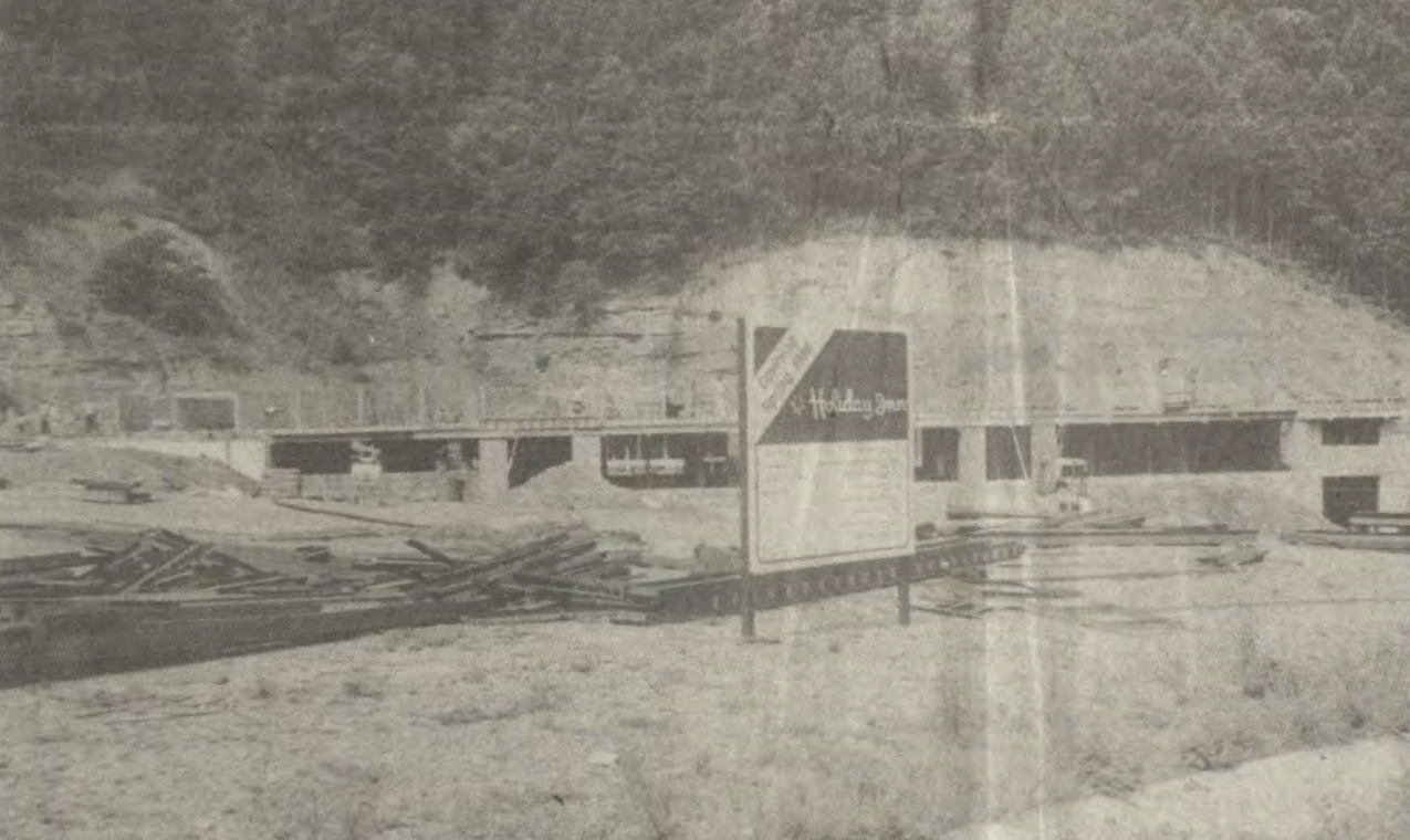
"OPENING SPRING, 1986," the sign says—and progress is apparent in the erection of the Holiday Inn on the outskirts of Prestonsburg. The rapid rise of the steel frame of the First Commonwealth Bank on Arnold Avenue and continuing work on Prestonsburg Village, the city's newest shopping center, are further evidence of a busy construction season here.
