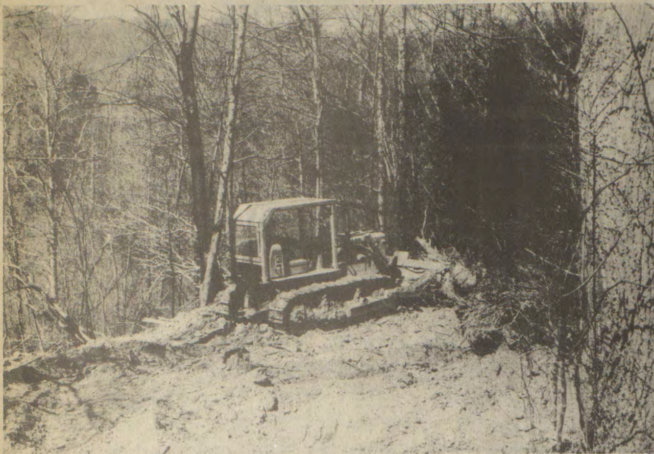
IN THE GERMAN BRIDGE AREA—a bulldozer cleans an area of trees and undergrowth at Camp Shawnee which is scheduled to open for school-aged children July 8 and last till August 2.
