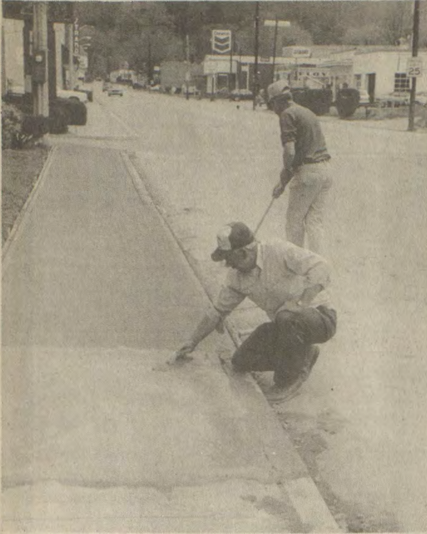
SIDEWALK WORK along Lake Drive near the center of town here is among the projects which the City of Prestonsburg is currently involved in, trying, like other communities around the county, to undo some of the damage of the past winter.
