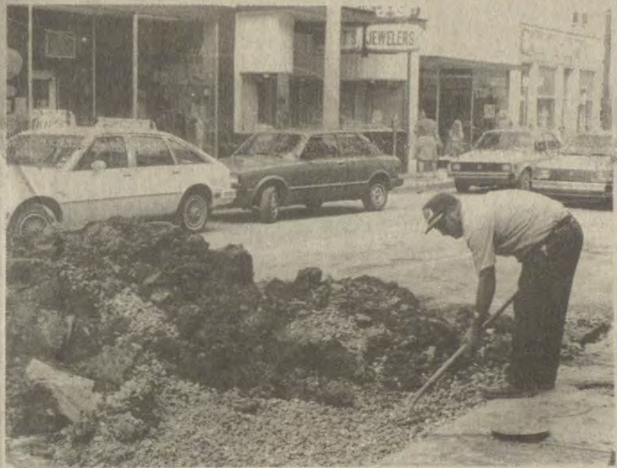
GETTING READY FOR RESURFACING of Court Street ran into considerable work for the Prestonsburg Utilities system and some disruption of traffic and business this week. The preparatory work included raising valve boxes and repairing sink holes, with excavation probing down several feet to water lines beneath the street.
