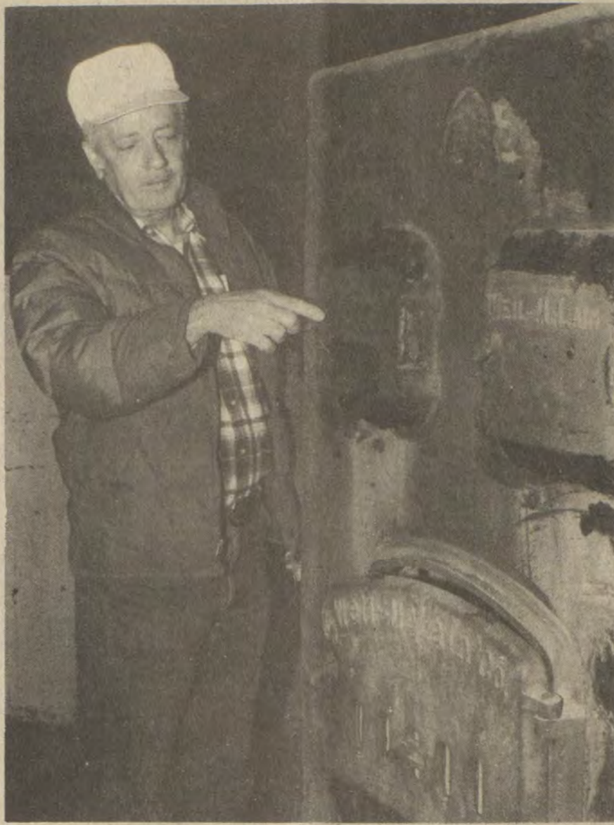
THE 30-YEAR-OLD BOILER at the McDowell School is "in excellent shape," although warped flue doors could have been the source of smoke which some say has bothered schoolchildren in nearby classrooms in recent years, said Aaron Miller, an inspector from the state fire marshal's office, following his inspection of the boiler last Thursday. The flue doors, to which Miller is pointing in the picture above, have been sealed pending their replacement.
