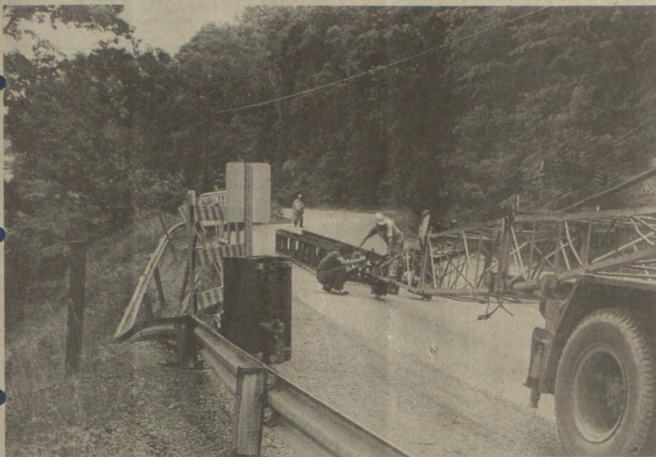
WORK BEGUN TUESDAY morning on an Abbott Mountain trouble spot should mean safer travel for the numerous motorists who daily cross the mountain on Route 1428. A state highway crew will attempt to fill where a section of the road near the top of the mountain slipped a number of years ago. Steel girders will be sunk into the underlying soil, according to a highways department spokesman, and reinforced guard rails will then be attached to the girders. The collapsed area of the roadway has been the site of several accidents over the years.
