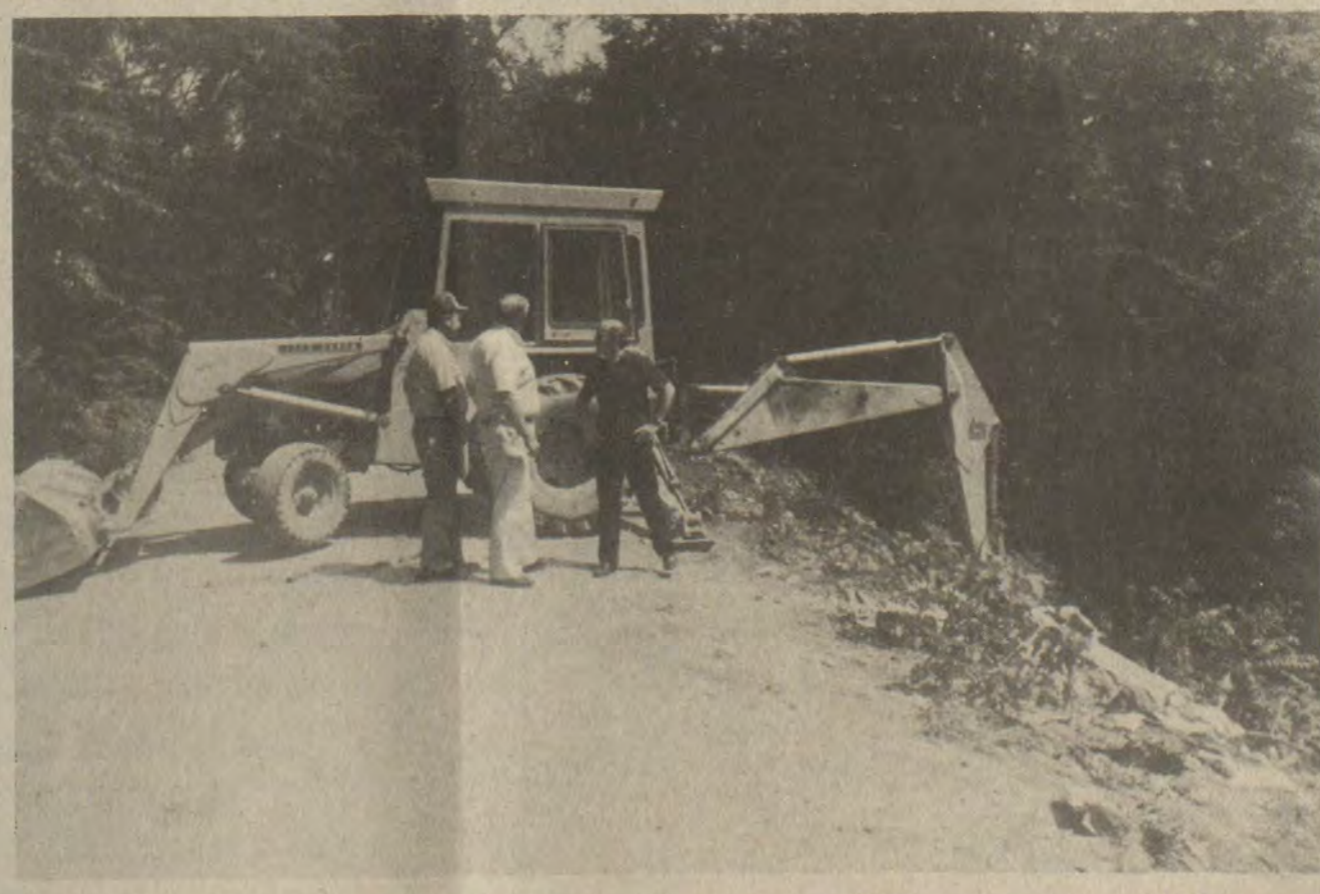
ROUGH AS IT IS, the road from East Point to Auxier is one of the area's most beautiful drives, particularly at the East Point end where a stand of fine beeches overlooks the town and the Big Sandy River. But it has also been the site for years of one of the county's most extensive and malodorous illegal garbage dumps.
