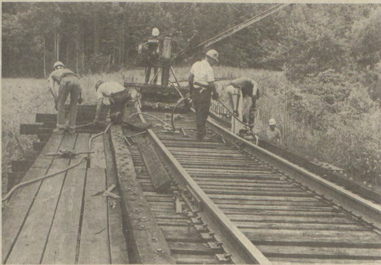
A WORK CREW over the weekend repaired blast damage done to a railroad trestle at Blue River, just upstream from the junction of the David road and Caney Fork of Middle Creek. A dynamite blast splintered the wooden structure late Friday night.
