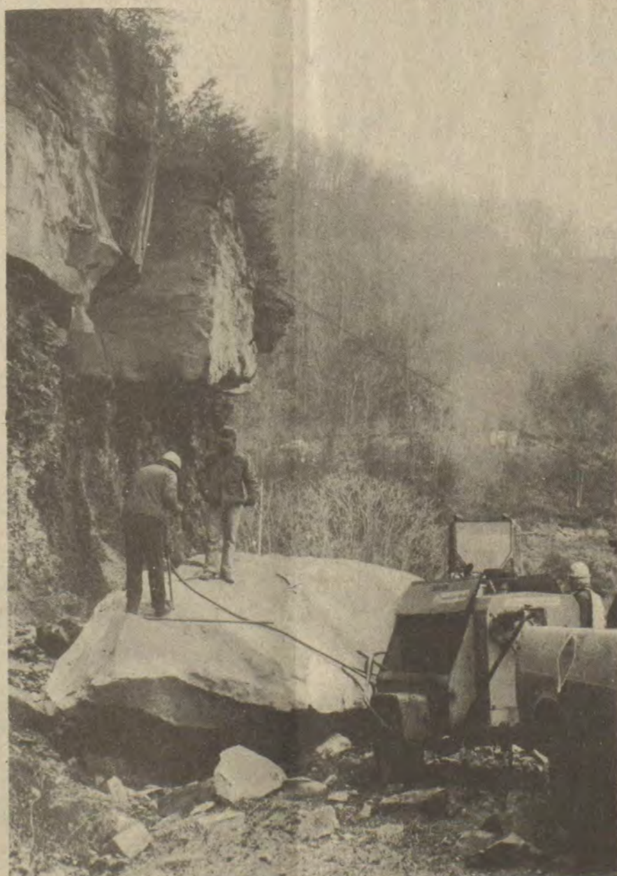
WORKMEN STILL LABORED Tuesday to remove rocks that tumbled from a highwall, spilling onto US 23, at Auxier day before. Boulders that fall periodically from the cliff face make the highway there a potentially perilous stretch, though no injuries were reported as a result of Monday's fall. Drilling into one monolith in an attempt to break it up are Dept. of Highways workers Ardrey Hamilton, left, of Teaberry, and Terry Tackett, of Drift.
