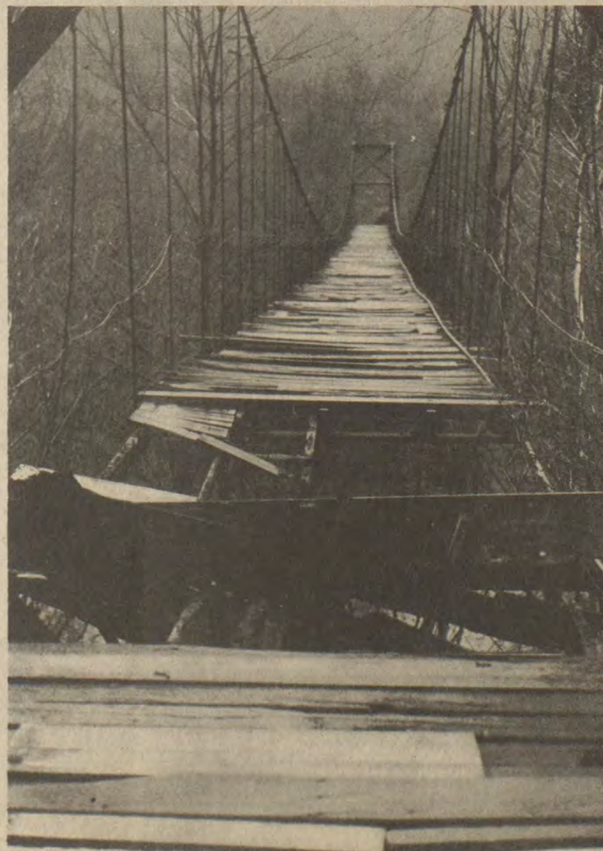
Photo shows where bridge section gave way, Saturday afternoon.
