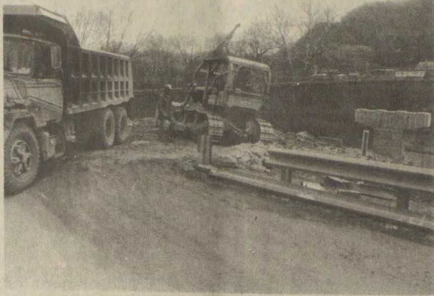
THE BOLDMAN BRIDGE, under construction since this summer, is not expected to be complete for a year. This week, however, pillars on which the new span will rest were complete, and loads of rock and dirt were being trucked. The wooden bridge which has served the community and a heavy flow of traffic for many years can be seen in the background.
