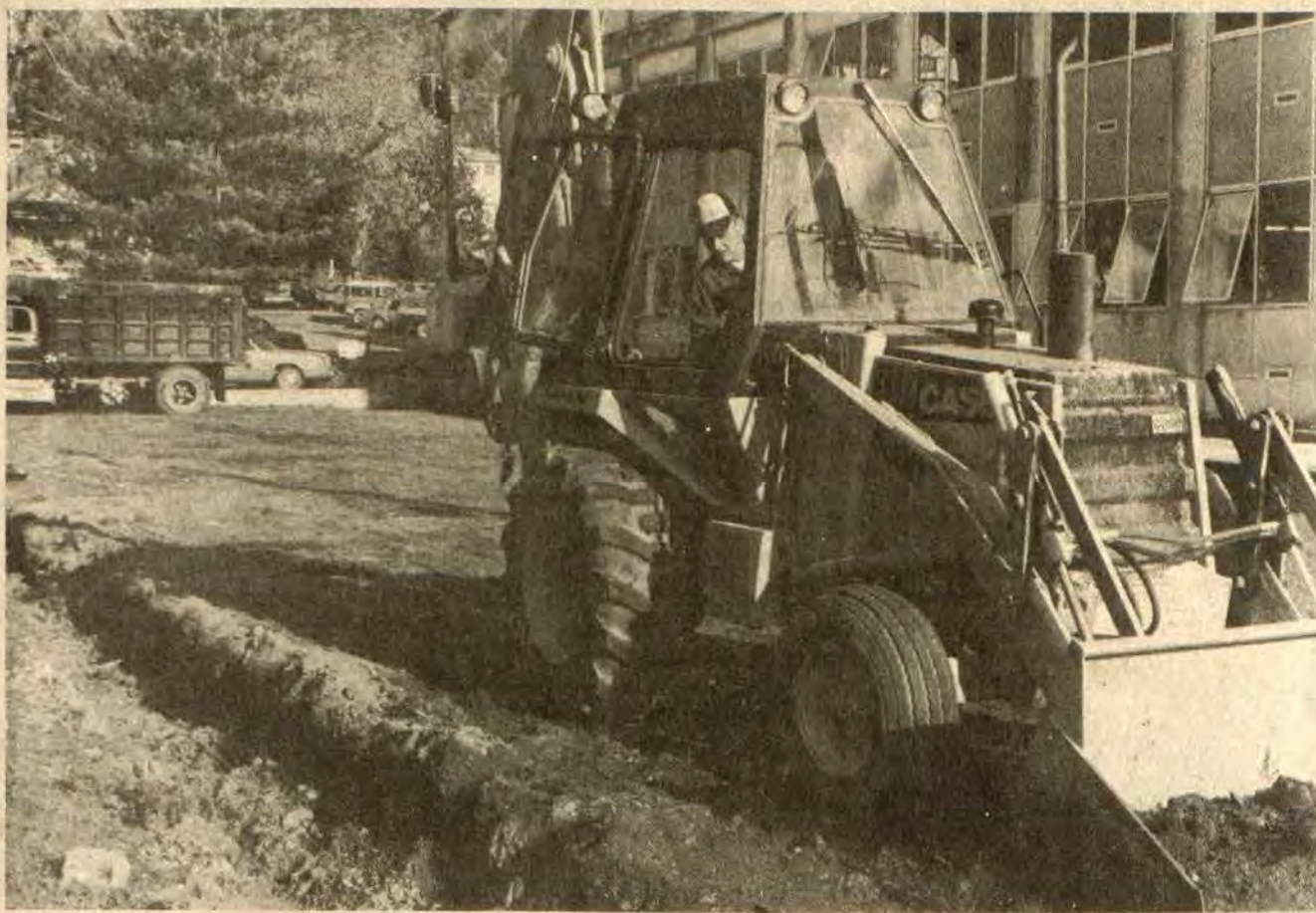
WORK WAS BEGUN over the past week to convert the area of lawn between the postoffice here and courthouse to a new parking lot to be used by employees and customers of the postoffice. It is hoped the work, which is being done by Witten Contractors, of Paintsville, will provide some relief to the frequent traffic snarls which have long plagued the intersection of Third and Court streets.
