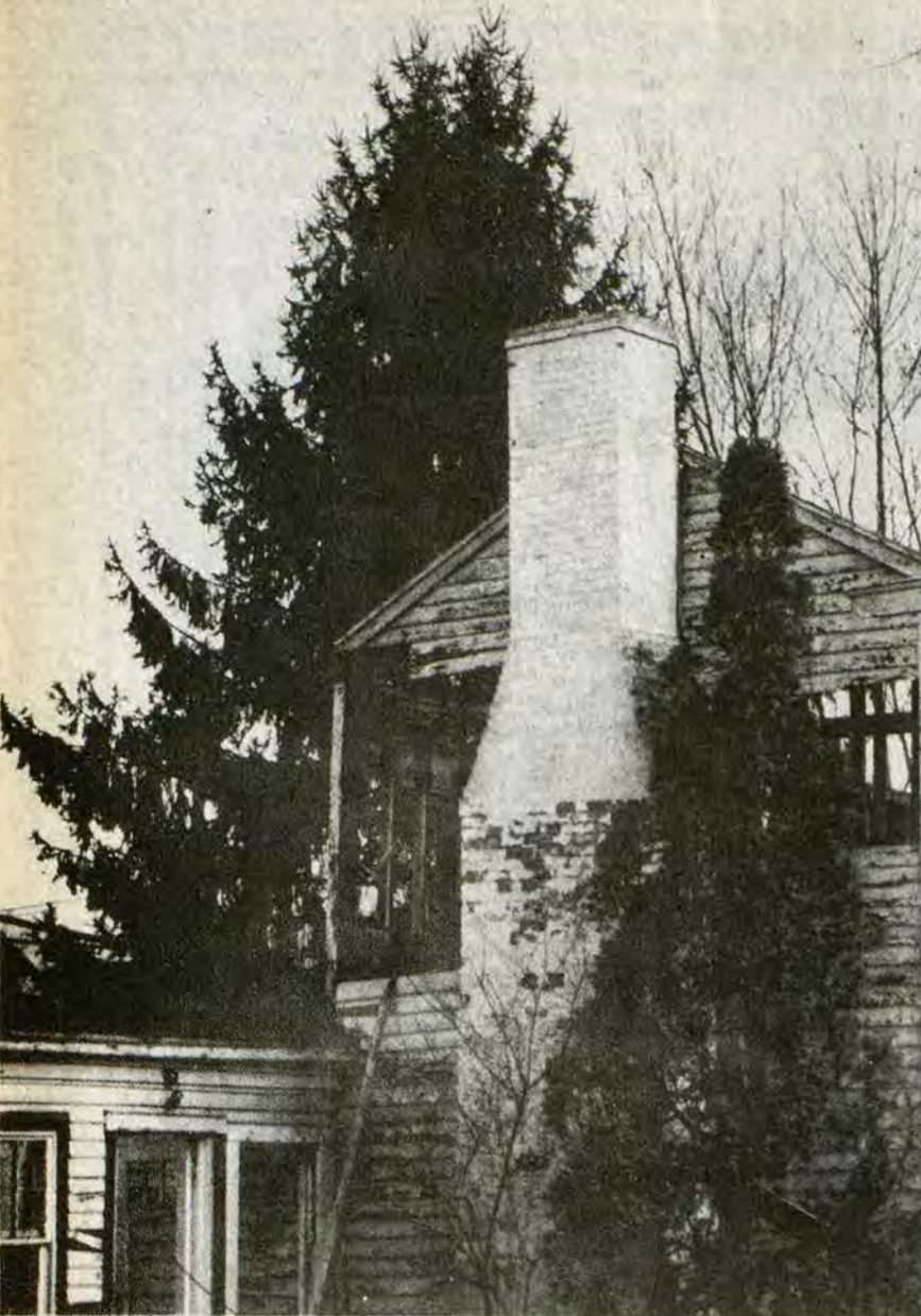
A VANISHING LANDMARK, the Civil War era Garfield Place here now stands in ruin alongside the ancient evergreens which dot the grounds. The historic structure is being razed to make room for future development.
