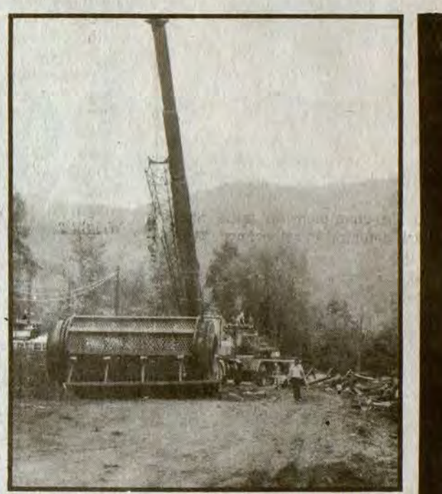
ROTARY BREAKER SYSTEM BEING INSTALLED BY SCALF ENGINEERING AT BELL COUNTY COAL CORPORATION, BELL COUNTY, KY.
