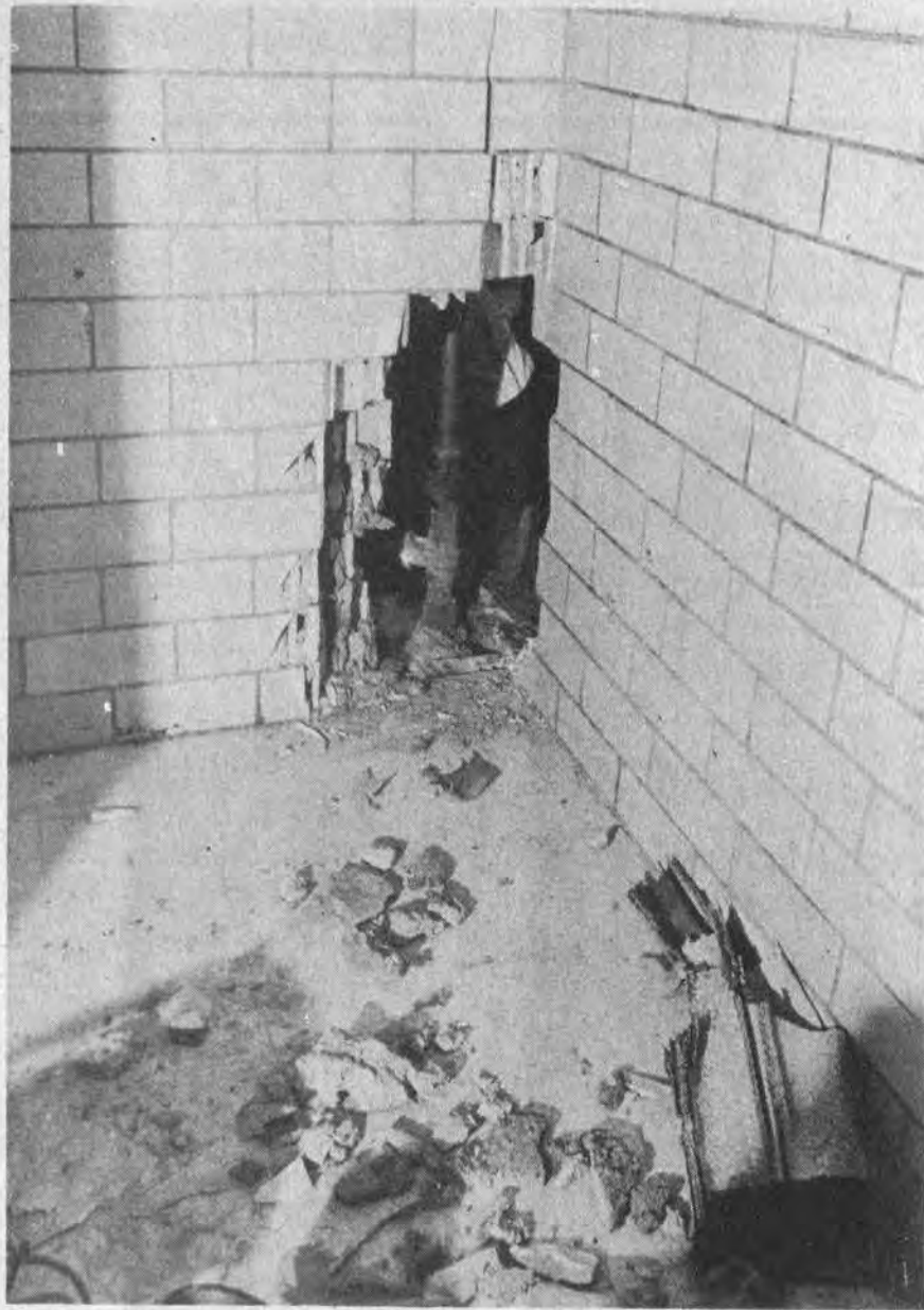
CHUNKS OF BLOCK and mortar litter the hallway outside boy's restroom at Prestonsburg high school where an explosion, last Wednesday morning, injured a PHS student and caused heavy damage. The blast blew an even larger hole through an adjoining classroom wall. (See story, Page 1.)
