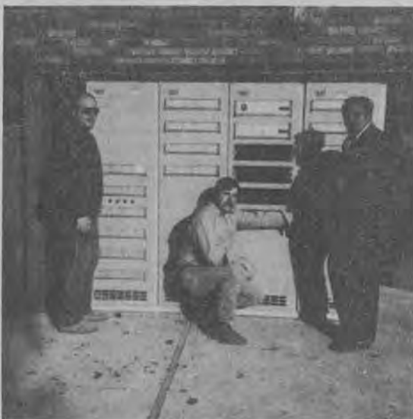
Pictured above is the head end equipment for the Martin tower located on a mountain peak approximately two miles east of the Floyd County town. From left to right are Paul D. Gearheart, Service Coordinator, Ralph Osborne, Head End Technician, and Charles Inglis, Chief Engineer.
