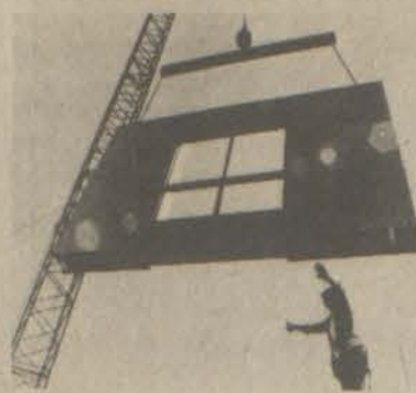
A workman gives the signal to "lower away" during installation of a U-Form at the Central Towers Apartments, a 232-unit HUD complex for the elderly in Detroit.
